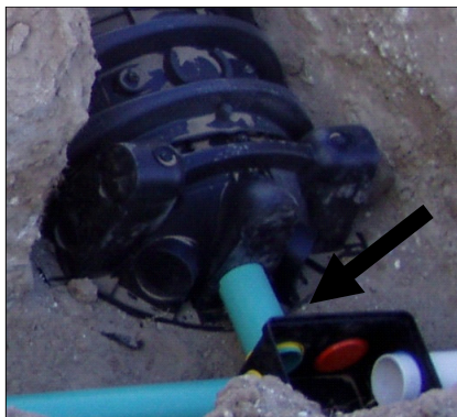
INCORRECT: BOTTOM PORT
